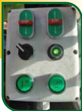
Comandi elettrici in cabina Electric controls in the cabin
